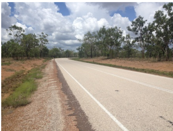
Plate 5 Kakadu Hwy - unsealed shoulders 190km from Jabiru
