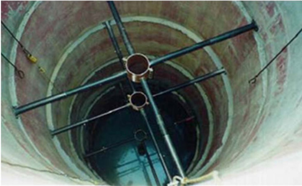
Figure 3-23: An example of a shaft pre-sink with raise bore pilot rod stabilisers
