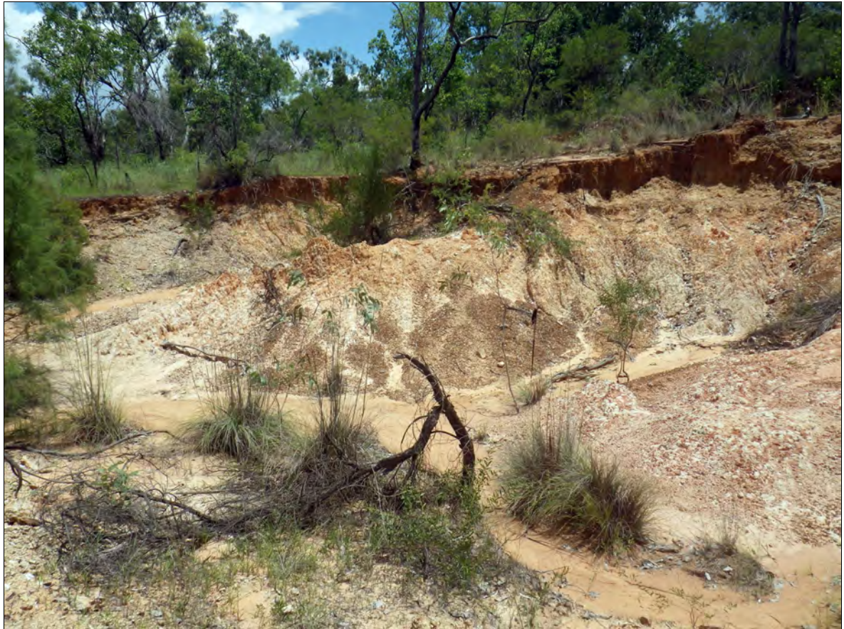
Figure 14. WDHRAS03 context view showing erosion gullies.
