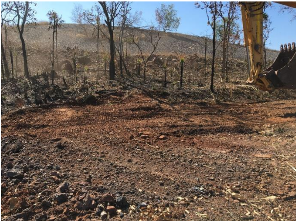
At WRTP-09 looking north at the southern batter of Dyson's Open Cut WRD
