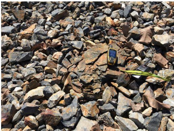
Deterioration of shale within dolomitic rock armouring
