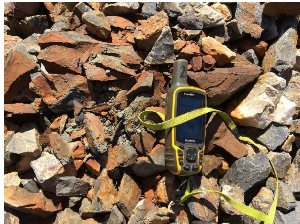
Close up of deteriorated shale within dolomitic rock armouring on Dyson’s Open Cut
