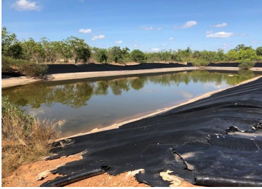
Stormwater pond, Rustler Roost
