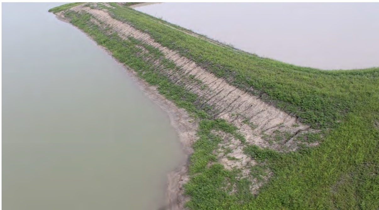
PLATE 5 EMBANKMENT WALL RILL EROSION, JANUARY 2017
