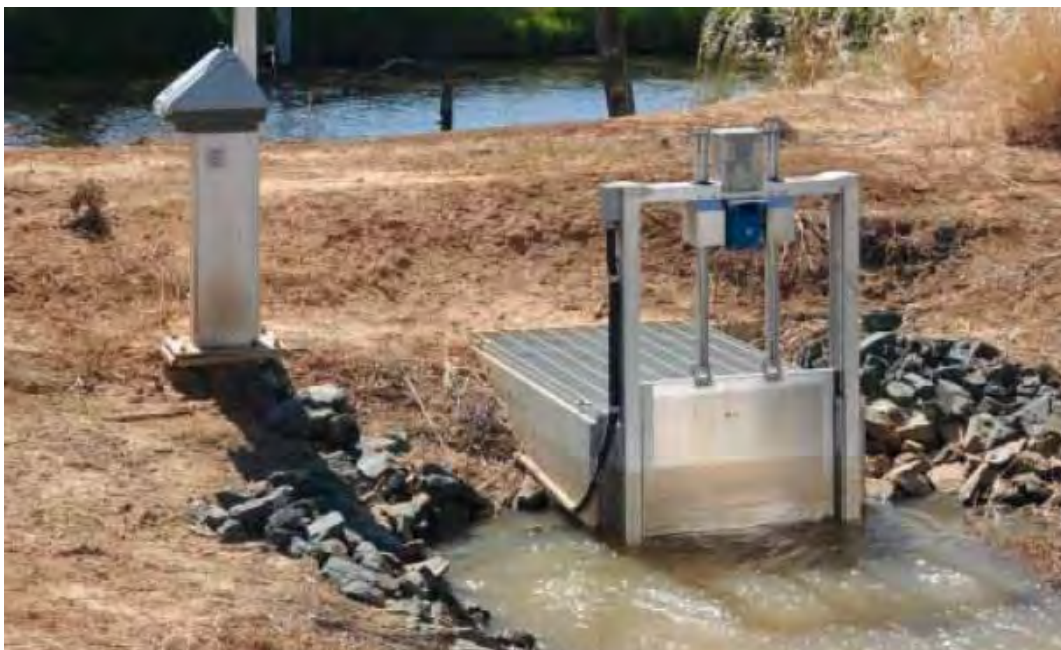
PLATE 10 EXAMPLE OF TYPICAL REMOTELY ACTUATED GATE
