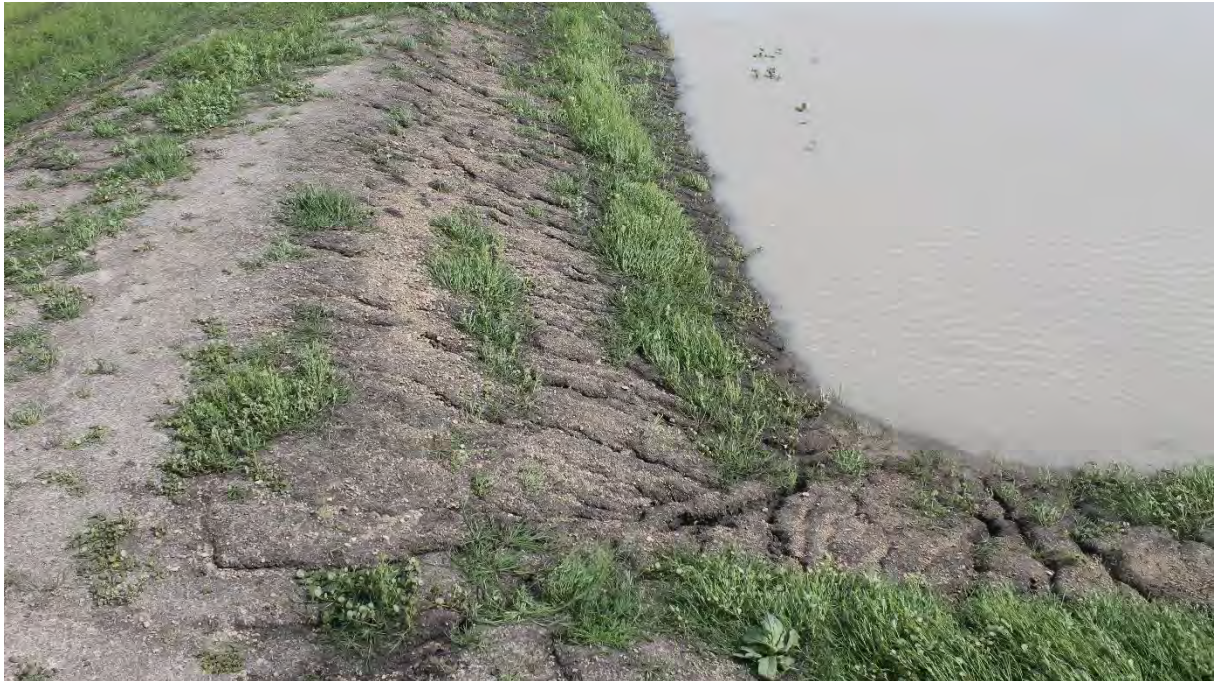
PLATE 7 EMBANKMENT WALL RILL EROSION, JANUARY 2017
