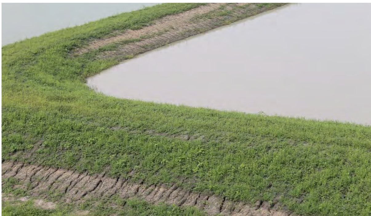
PLATE 6 EMBANKMENT WALL RILL EROSION, JANUARY 2017
