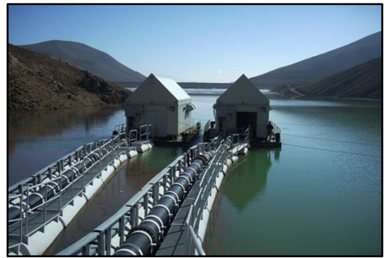
Photo 2: Photograph showing typical barge decant and pontoon arrangement.
