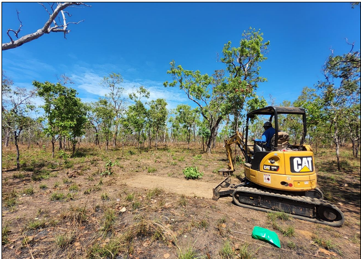
Figure 1: View of central area of the site at test pit 16, with 3 tonne excavator.
