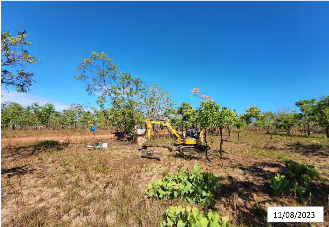
Photo 5: Near Test Pit 41, showing airport road, which runs through the site and natural bush either side, minor litter.
